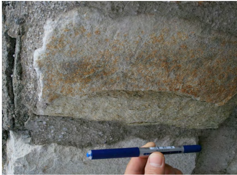
Figure 4 Deterioration in restored stone
