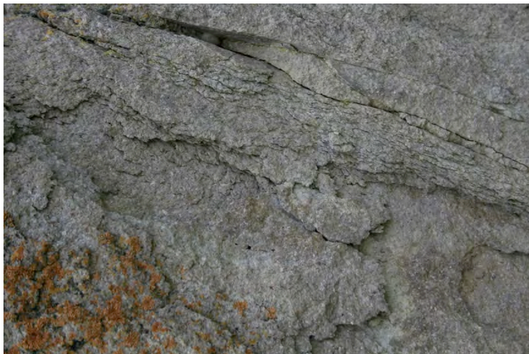
Figure 5 Deterioration in natural stone forming the base of the castle
