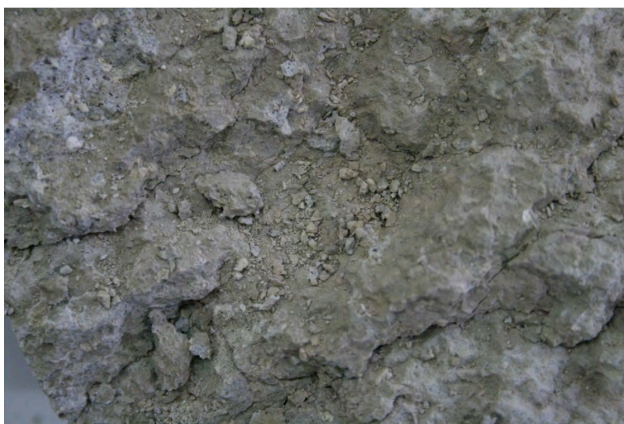
Figure 11 Deteriorated and flaked surface of Stone 5
