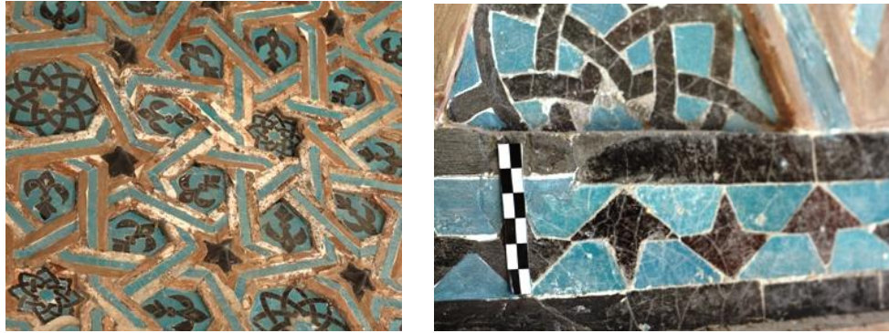
Figure 3.2 North Eyvan wall and dome. Painted imitation tiles were detached and the original ones were not differentiated by eye.
