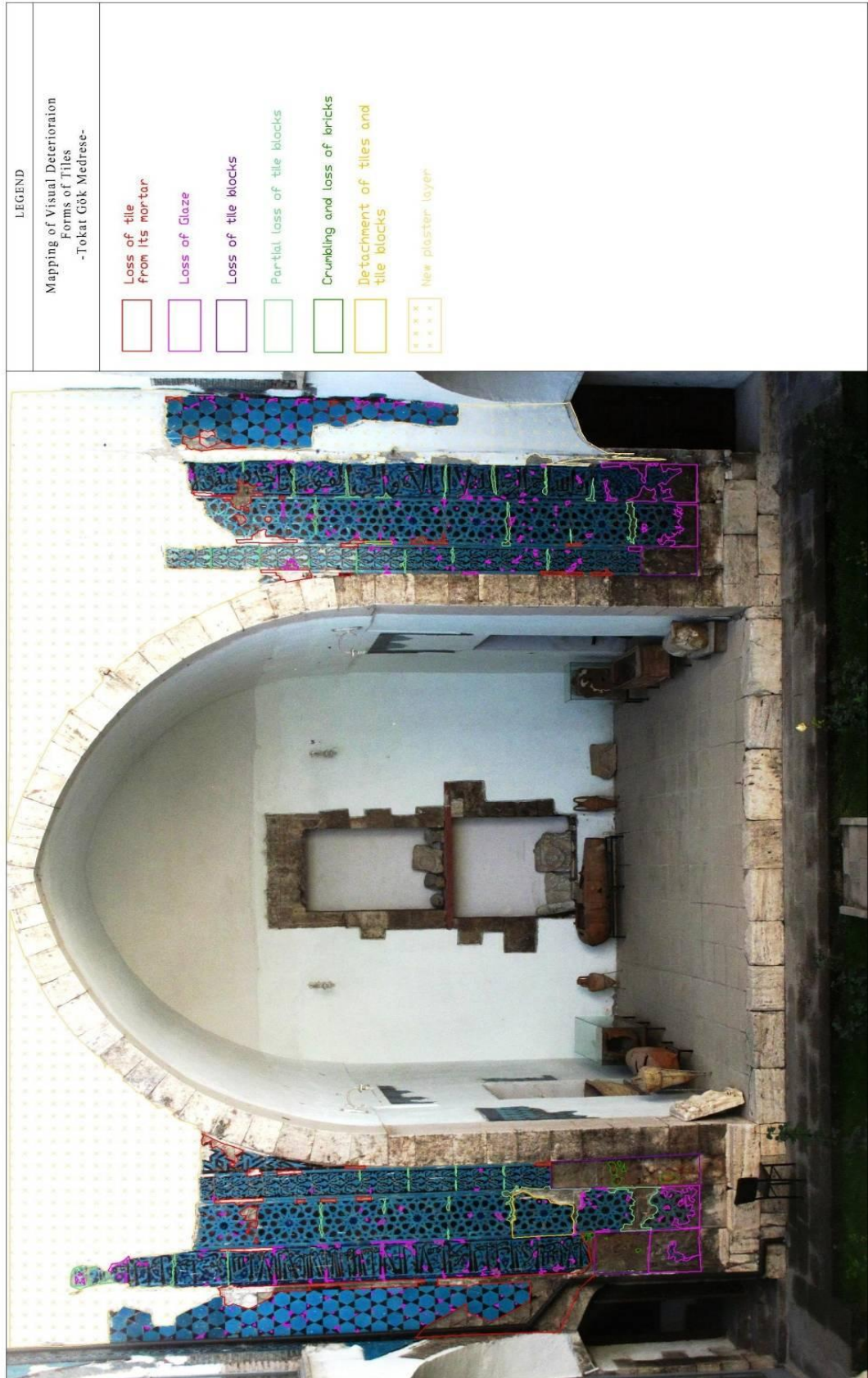
Figure 4.3 Mapping of visual decay forms in Tokat Gökmedrese
