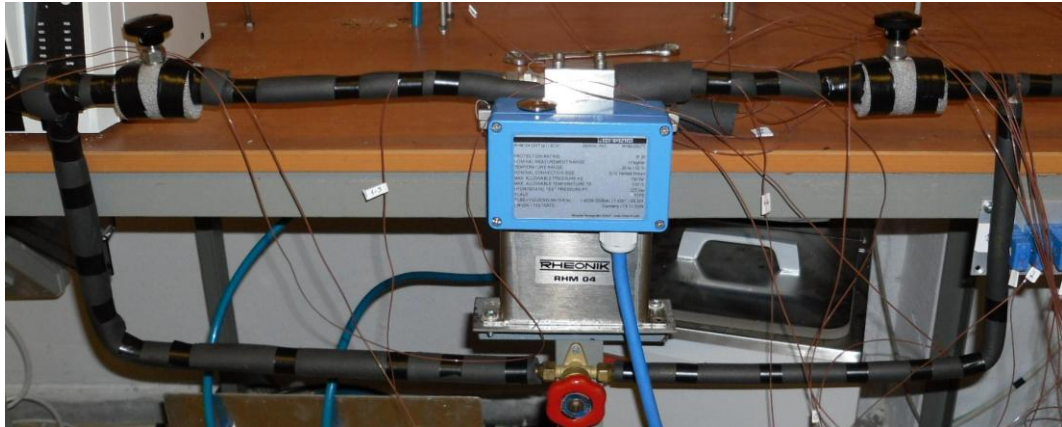
Figure 8: The flowmeter and by-pass line
