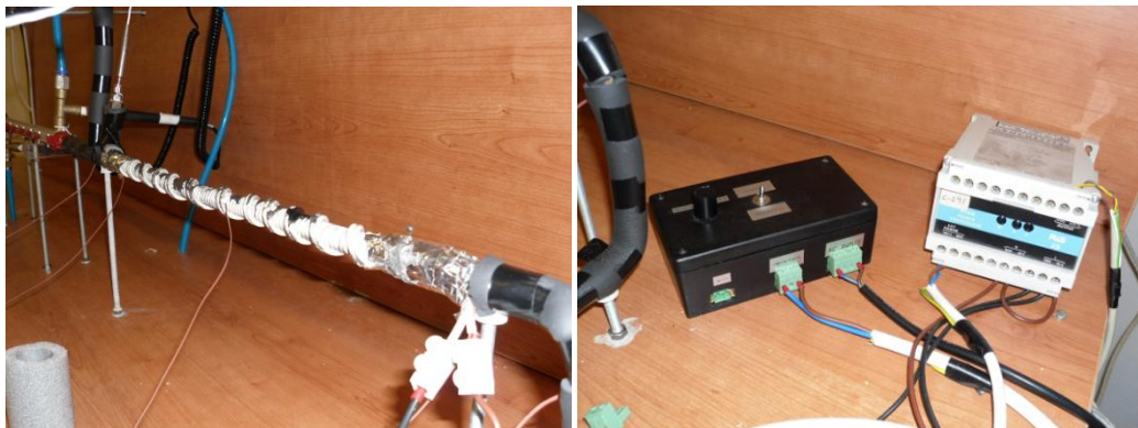
Figure 6: The pre-heater without the insulation, the control box and the power transducer
