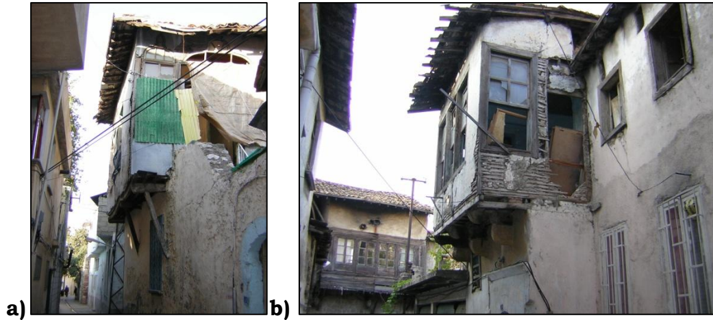
Figure 3.49. a) A traditional house in Özdemir Street: An example of a personal attempt to repair an original window (Photograph: Rifaioğlu, M.N., 2005) b) A deteriorated and vacant traditional house in Sokullu Street (Photograph: Rifaioğlu, M.N., 2005).
