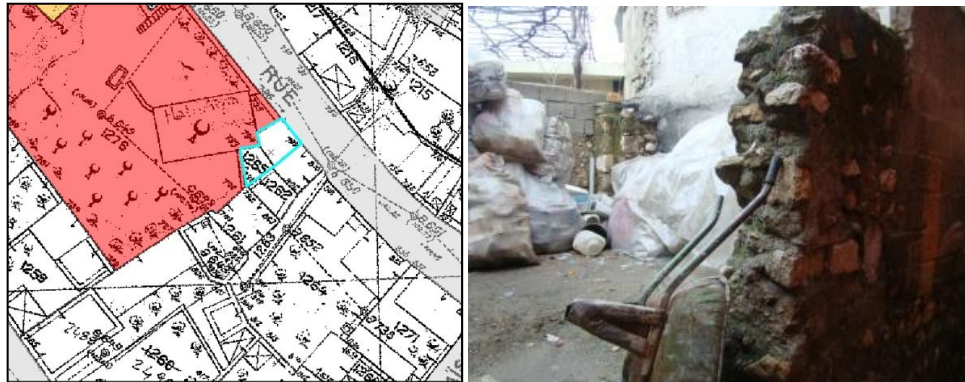
Figure 4.100. A demolished single room-dwelling owned by a Mosque foundation (Photo: Rifaioglu, M. N., 2009)
