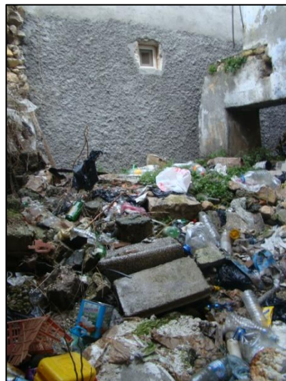
Figure 4.98. A ruined one-room dwelling located at the end of a private cul-de-sac (Photos: Rifaioğlu, M. N., 2009)
