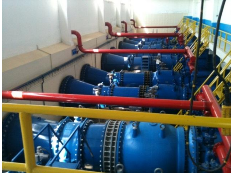
Figure E.2 Pipelines entering İvedik WTP
