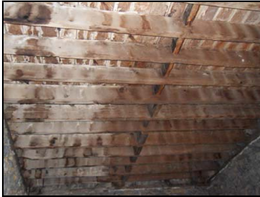
Figure 2.58. Timber girder floor of space E07 and E08, view from space G01
