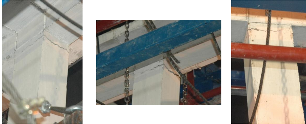
Figure 2. 16: Damage observations from 3 rd Story Columns (SP3)
