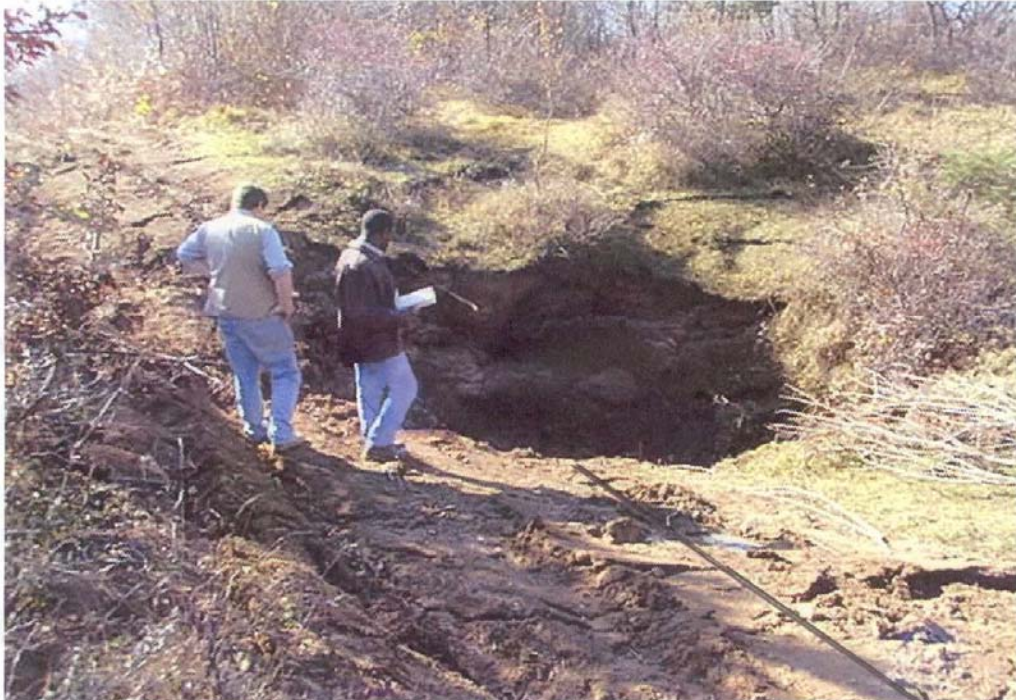
Figure 3.17 Sinkhole formed due to Bolu Tunnel collapse at Elmalık Right Tube (after Yüksel-Rendel Engineers, 1999)
