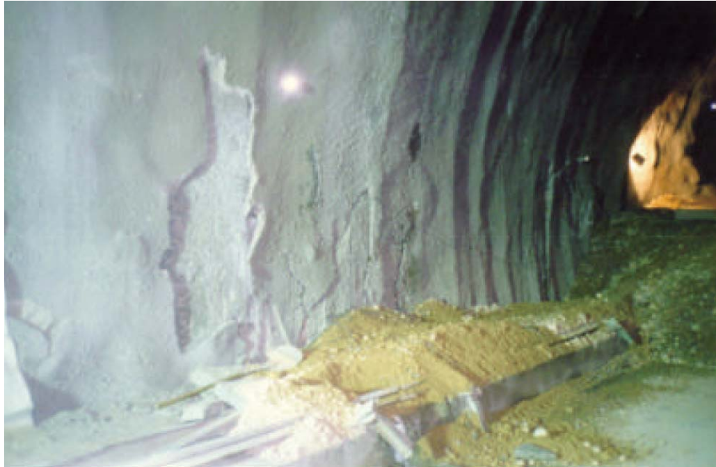
Figure 3.18 Spalled shotcrete liner segment (after Ghasemi et al., 2000)
