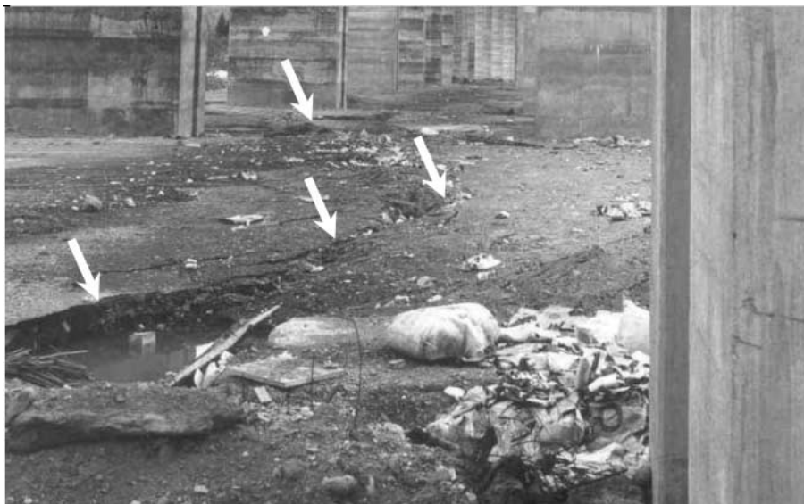
Figure 3.8 Fault rupture (indicated by arrows) crossing through the viaduct piers. Courtesy G. Macchi. (after Faccioli et al., 2002)
