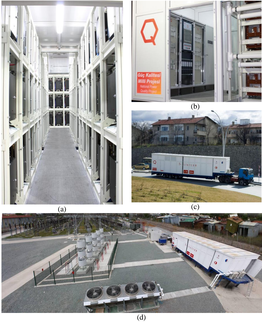
Figure 5.2 154 kV, \pm 50 MVar T-STATCOM based on 11-level CMC installed at 380kV/154kV Sincan Transformer Substation ((a) Interior view of trailer with power stages, (b) Control cabinets, (c) Trailer for \pm 50 MVar T-STATCOM on road (WxLxH:3700mmx16800mmx4300mm), and (d) General view of T-STATCOM)
