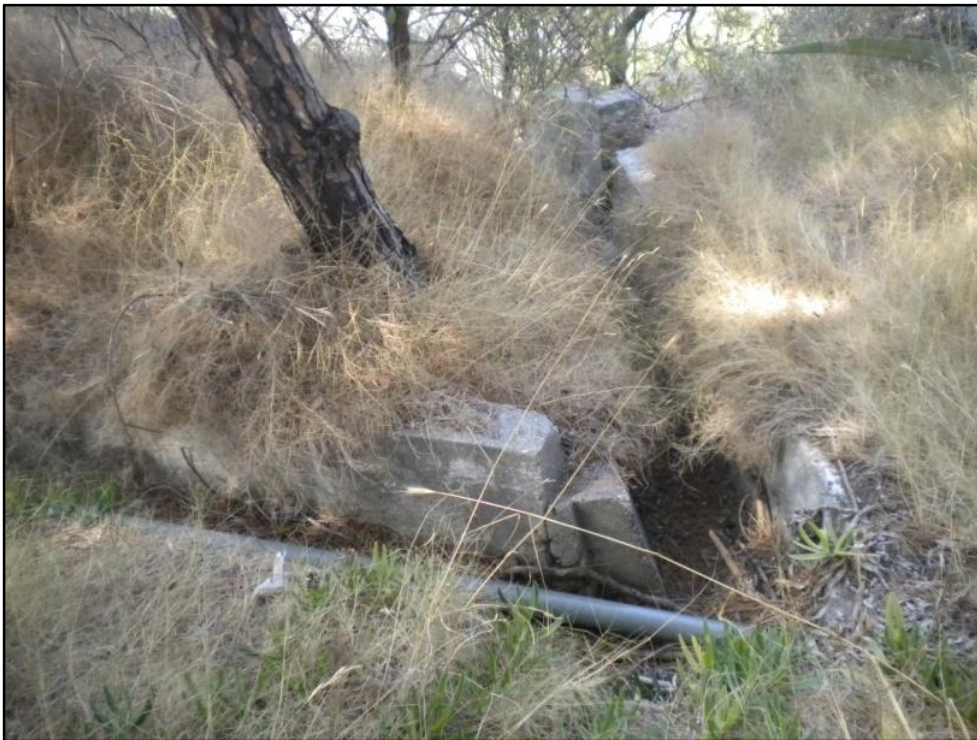
Figure 5.2 Improper installation of the old drain line.
