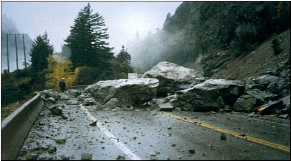
Figure 2.2 Highway closure caused by rockfall in very strong, blocky granite from a height of about 300 m (Dorren, 2002).
