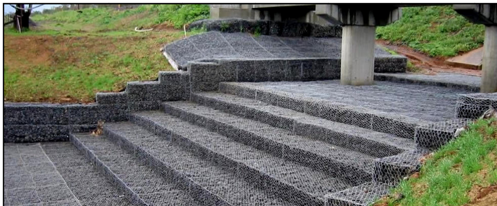
Figure 3.8 Use of gabion mattress as scour countermeasure at a bridge location ( http://www.tradekorea.com/sell-leads-detail/S00025110/Gabion_Mattress.html , 2012)
