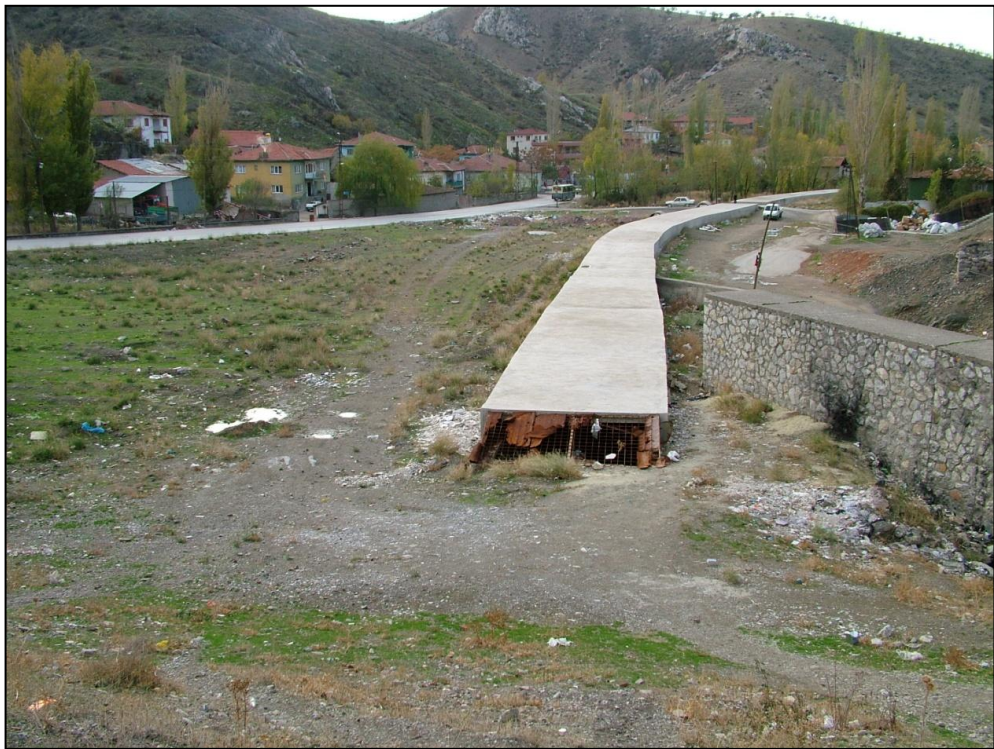
Figure 3.42 Closed Conduit at the exit of İncesu Detention Pond (DSİ, 2008)
