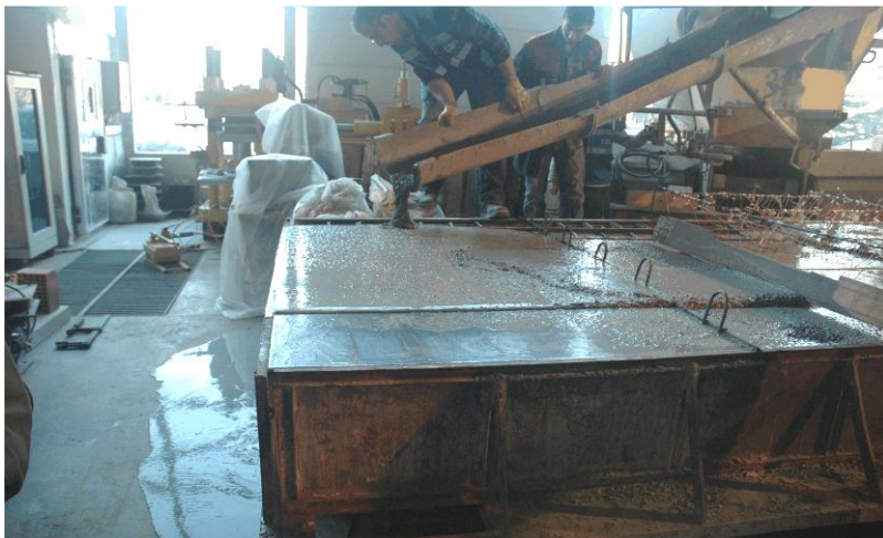
Figure 3.1 Bleeding observed during pouring of concrete
