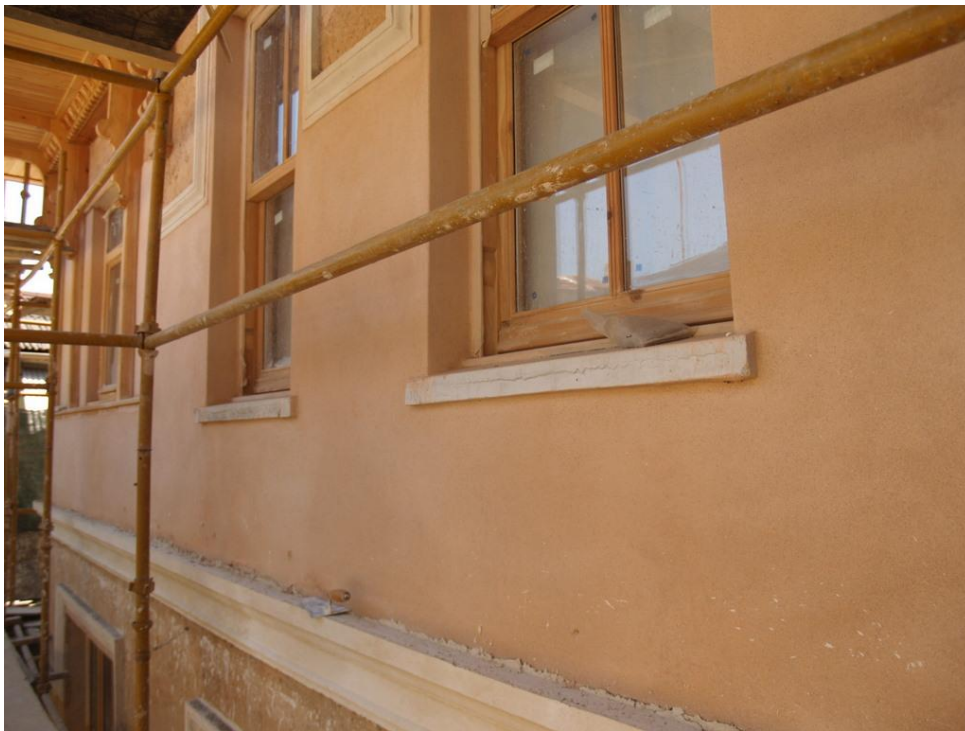
Figure 64: Sills and window sills of Building on Block 2307 Lot 28 during restoration (Altınsay Özgüner, 2009)
