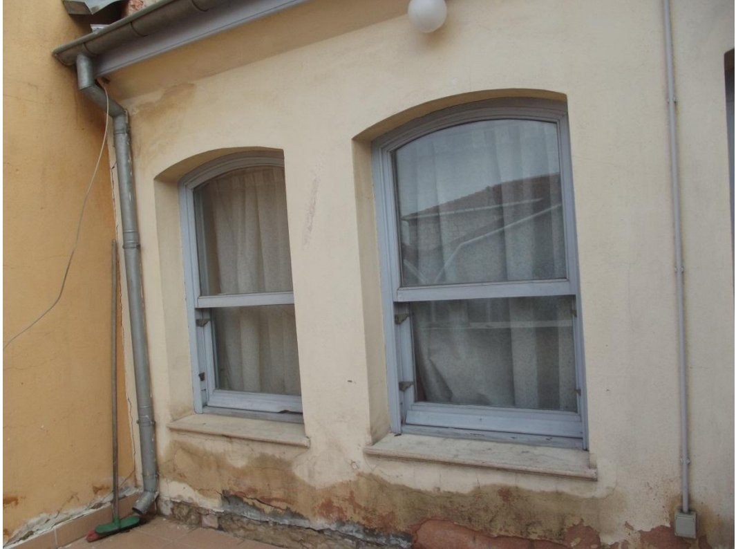
Figure 77: Dampness problem in the terrace
