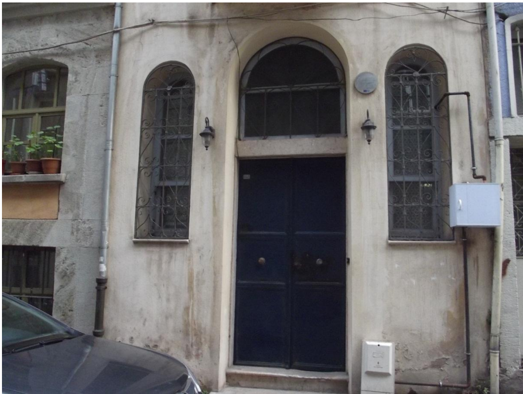
Figure 76: Dampness problem on the facade
