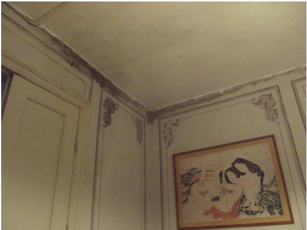
Figure 78: Deterioration in ceiling
