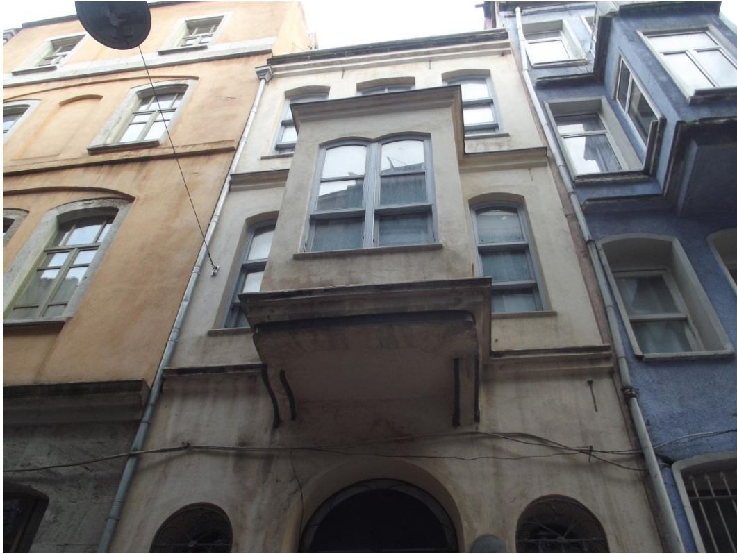
Figure 75: Stains on facade
