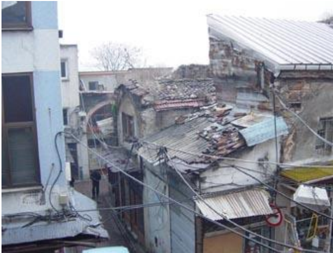
Figure 58: Condition of Fener Balat houses (Altınsay Özgüner, 2009)
