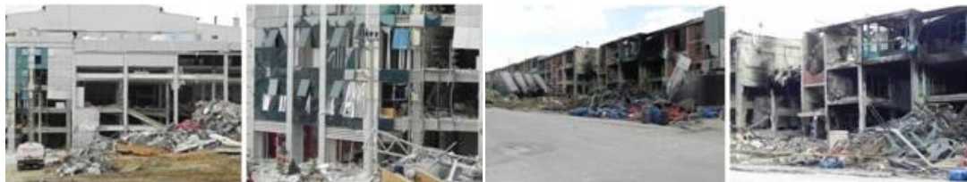
Figure A.9: Industrial facility explosions in Ankara. In the OSTİM region; two separate buildings exploded on the same day (of February 3, 2011). Beside the extensive damages on the buildings, totally 20 workers were killed in both facilities. Pictures are from Ali Tolga Özden's archive (2011).
