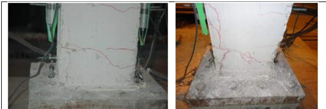
Figure 2. 14 Reinforcement pullout at spliced regions (SP2)
