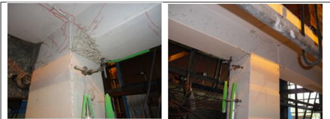
Figure 2. 12 Damage observed at peak displacement (SP2)
