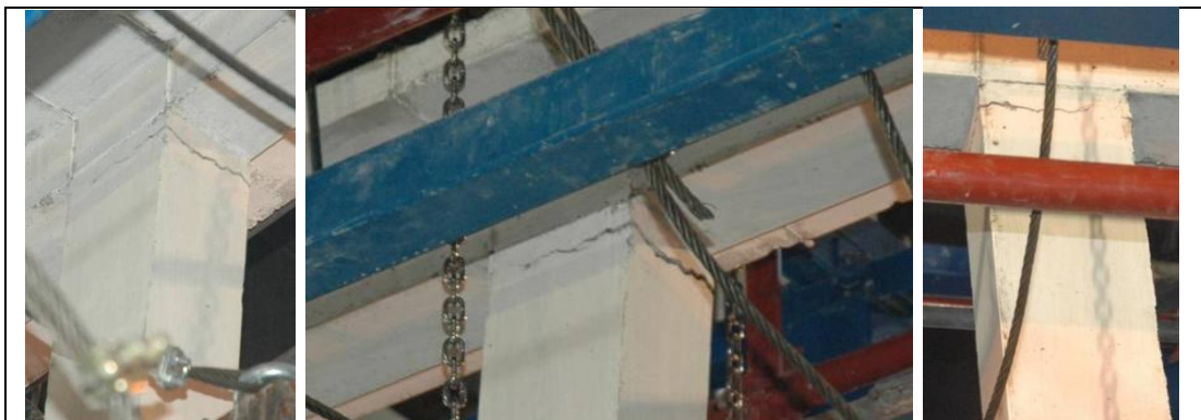
Figure 2. 9 Damages observed in the 3 rd storey columns (SP1)
