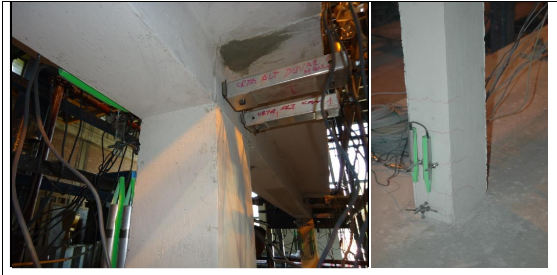
Figure 3. 21 Specimen #2 1 st storey column damages during D2
