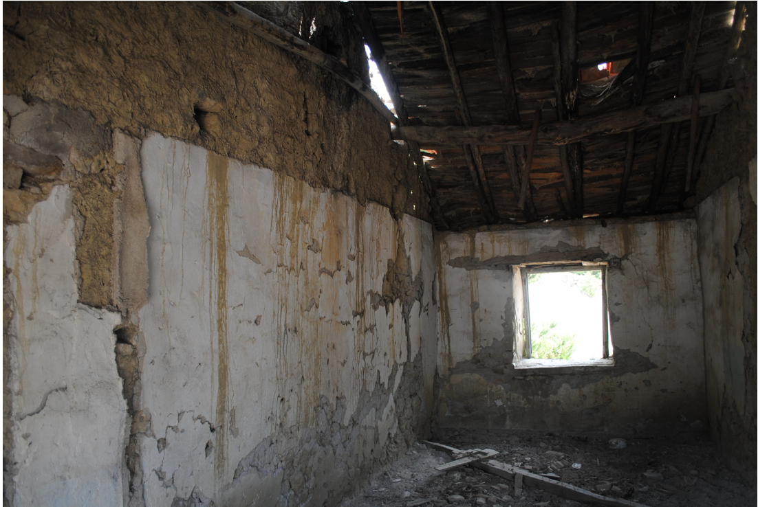
Photo. 66: Interior of the school. Note the mud-plaster, whitewash and the timber roof structure.
