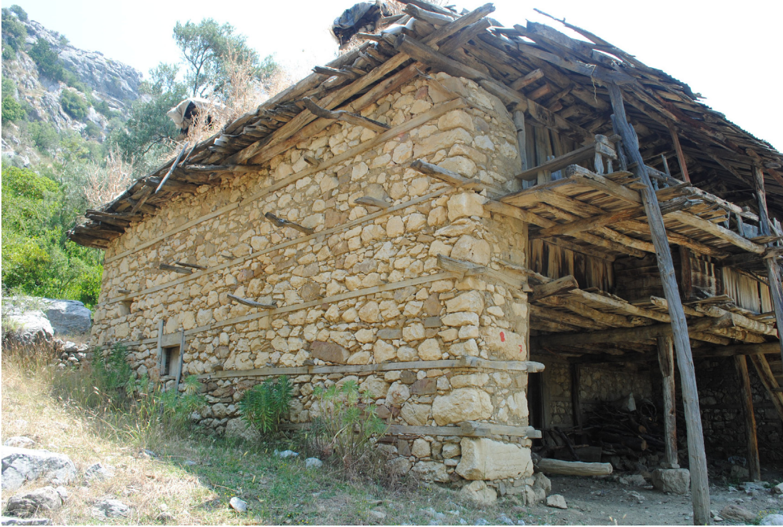
Photo. 64: A typical rubble wall construction. Note the load distributing timber beams evenly spaced between rubble courses.
