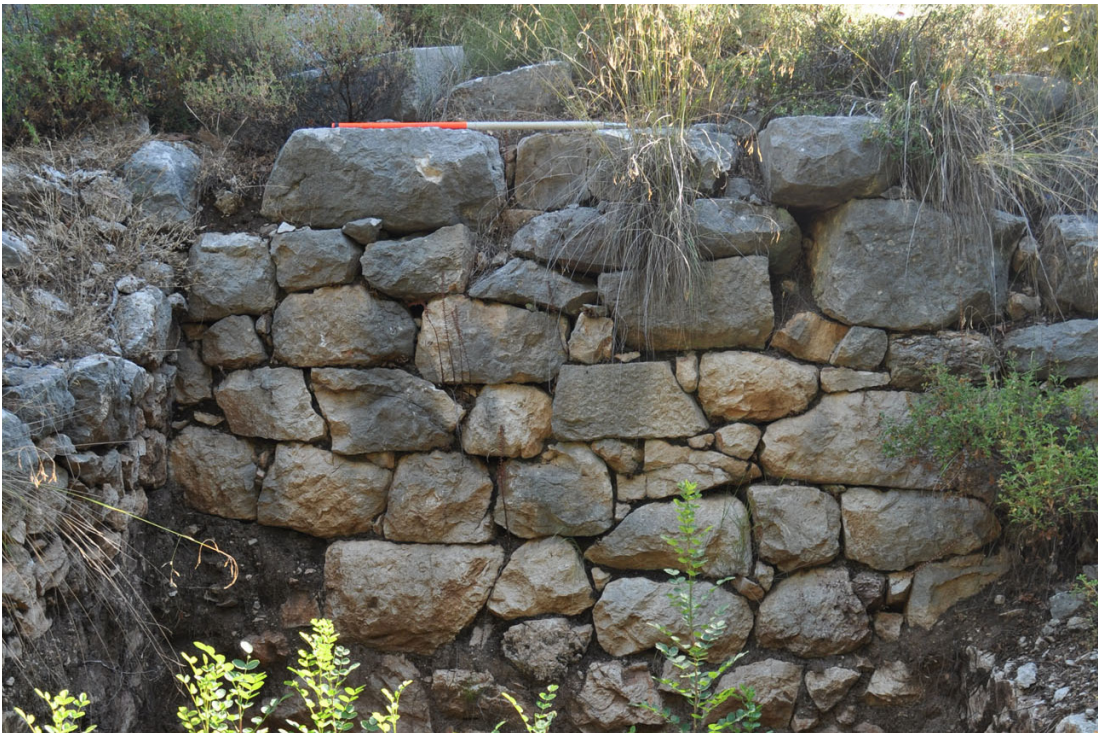
Photo. 24: A typical stretch of a terrace wall exposed by treasure hunters.
