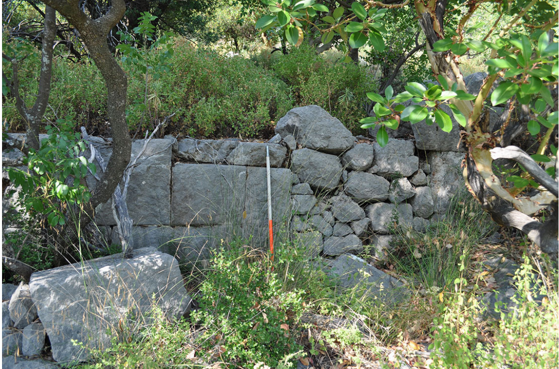
Photo. 59: An example of a later modification in a dwelling. Existing doorway in a facade made of cut stone blocks is blocked with rubble infill.
