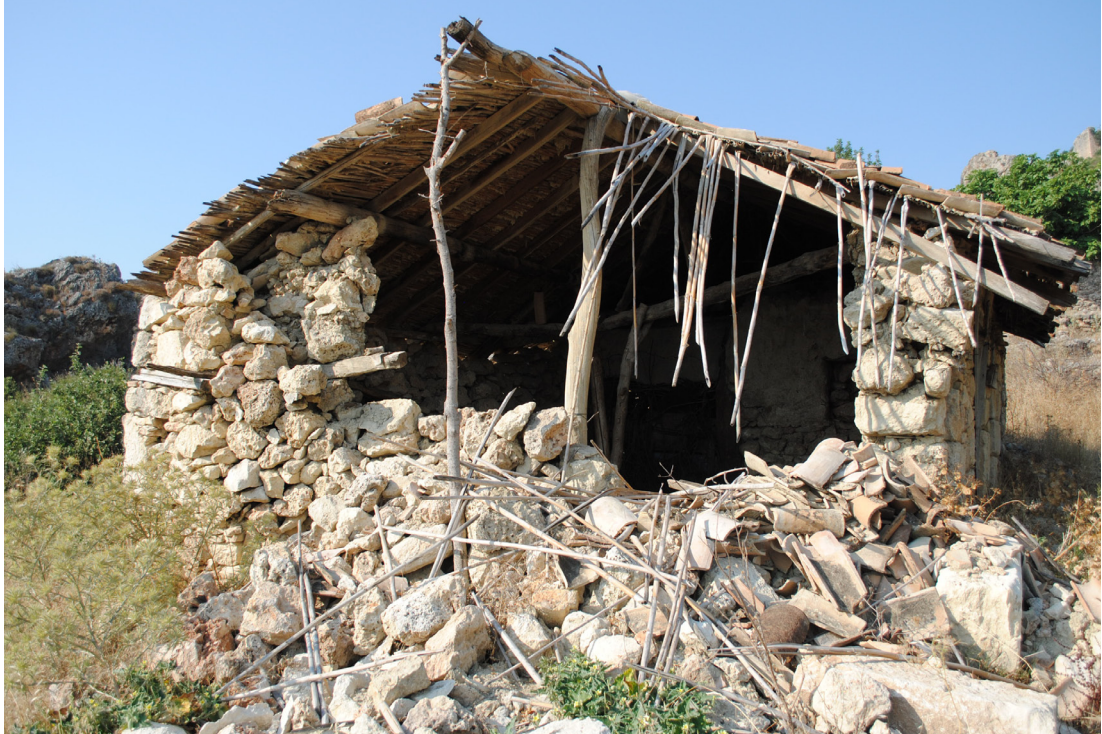
Photo. 67: Reeds have been used as an underlayer beneath ceramic roof tiles. Also note the plaster and whitewash use on interior wall faces.
