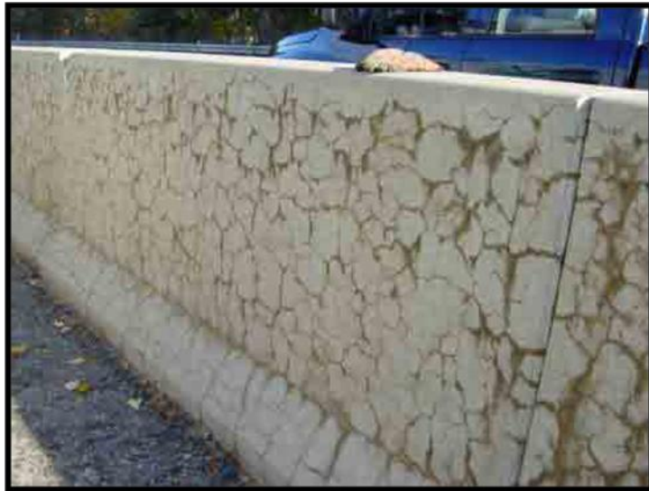
Figure 2.2 ASR Cracks on Concrete Step Barrier [FHWA, 2010].
