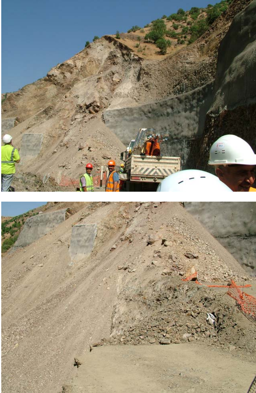
Figure G.1 Çetin Dam and HEPP Diversion Tunnel Outlet Incident
