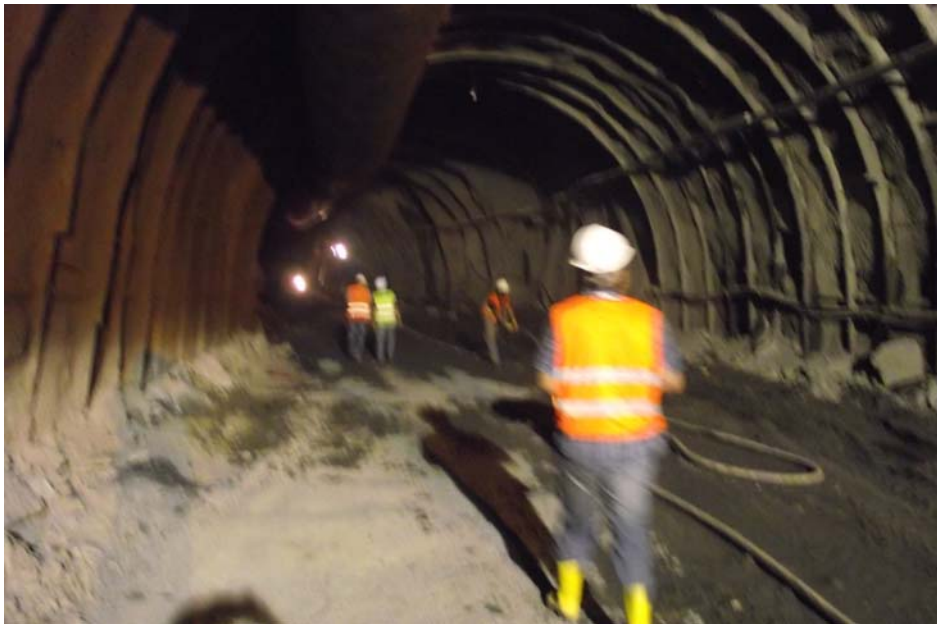
Figure H.2 Workers Wearing Safety Clothes at Çetin Dam and HEPP Diversion Tunnel
