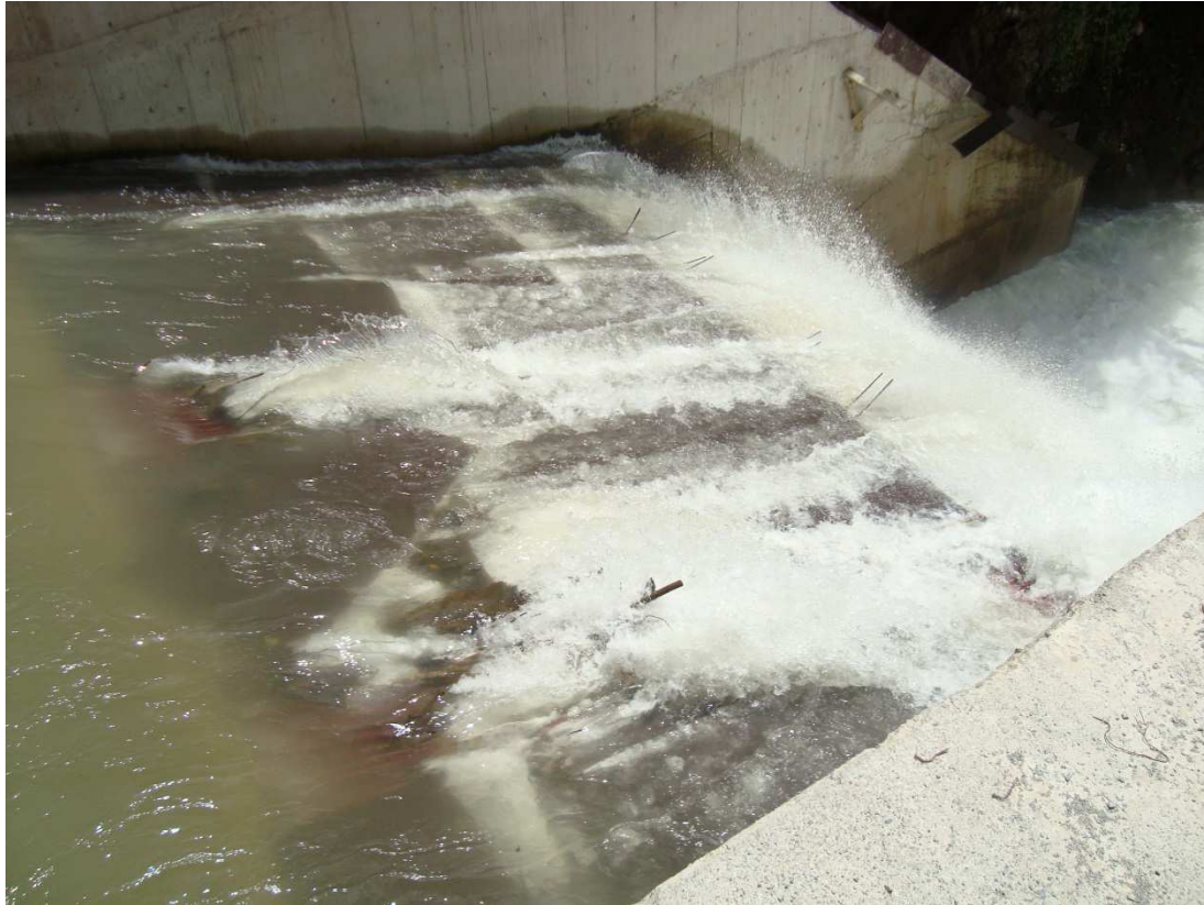
Figure 55 : Trash rack of Arpa Weir and HEPP
