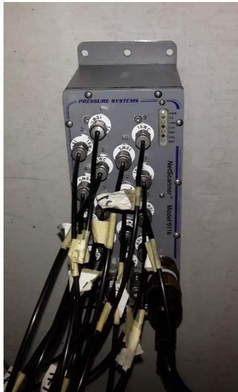
Figure 3.13 The 16-channel pressure scanner system used in the experiments
