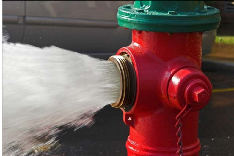
Figure 2.1 : Fire Hydrant Flushing (Web 1)
