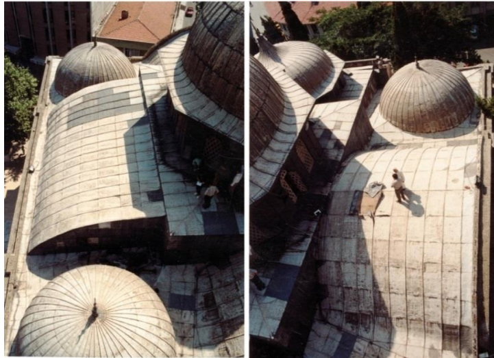
Figure. 122 The cover structure of Balıkesir Zağnos Pasha Mosque. On the left the half barrel vault and two small domes on the north part is seen. On the right, the vault and the small dome is seen. Source: VGM Archive, retrieved in 2011
