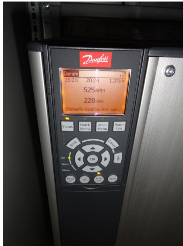
Figure 4.6: Indicator of control panel
