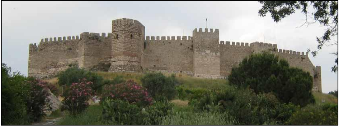
Figure 3-31 Southern side of the Inner castle before and after the strengthening of the walls (personal archive)
