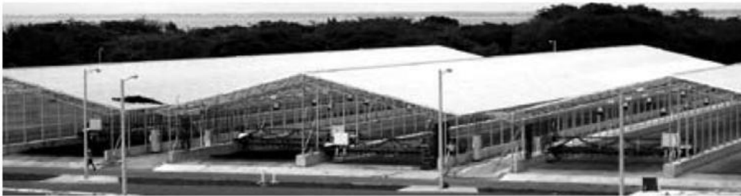
Figure 2.10 A view of the solar sludge drying plant in Managua/Nicaragua (Scharenberg et al., 2010)
