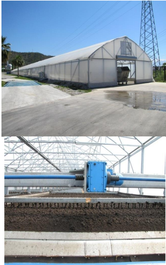
Figure 2.12 Fethiye Waste Water Treatment Plant Greenhouse Solar Drying Unit (April, 2013)
