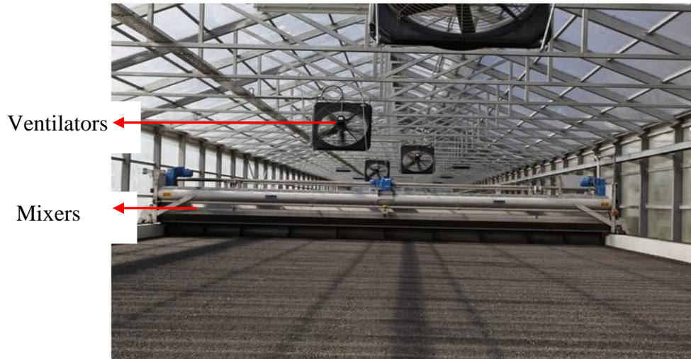
Figure 2.13 A greenhouse solar dryer system by Huber (URL 14)
