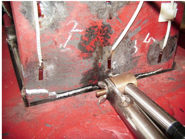
Figure 7.4. Front view of fracture occurs exactly above the 400 mm-high steel base fixture.
