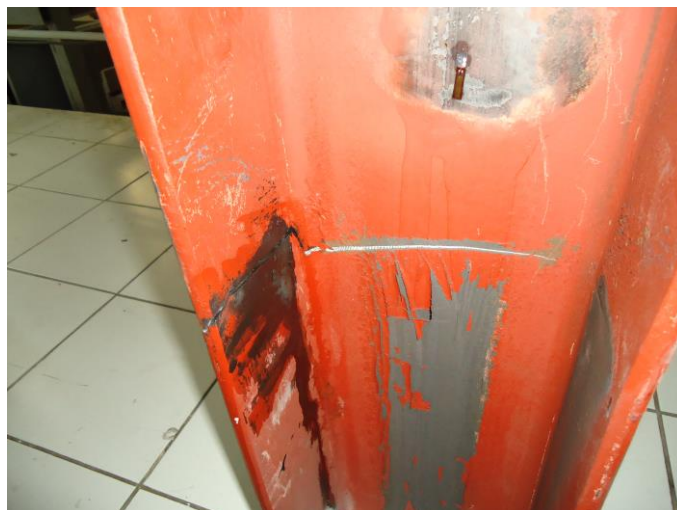
Figure 7.16. Fracture occurs on flange and web above the 400 mm-high steel base fixture.
