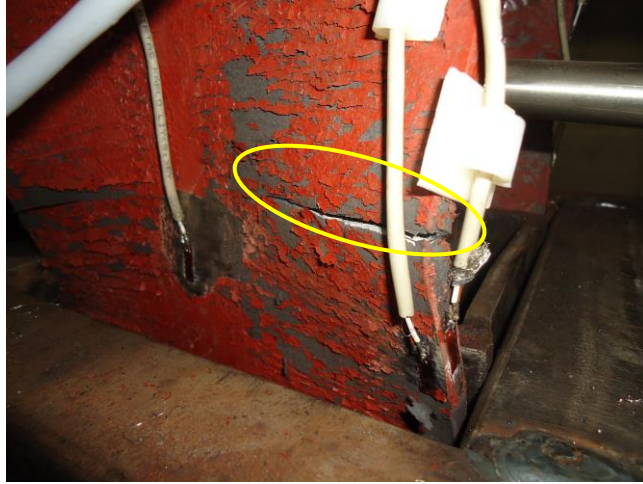
Figure 7.52. Close view of the crack.
