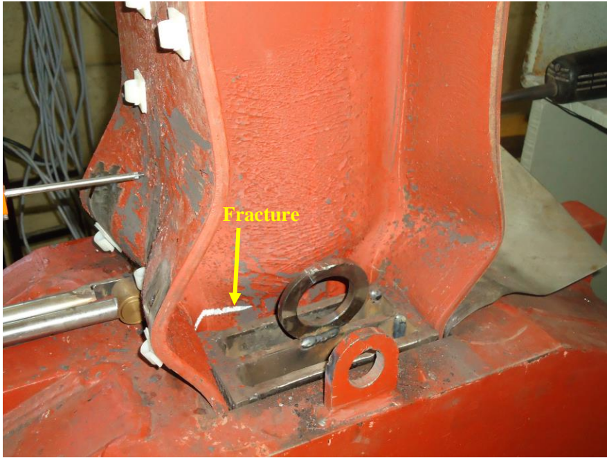
Figure 7.44. Fracture occurs on web.
