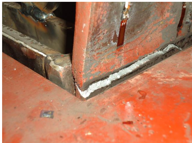
Figure 7.11. Front view of fracture occurs exactly above the 400 mm-high steel base fixture.
