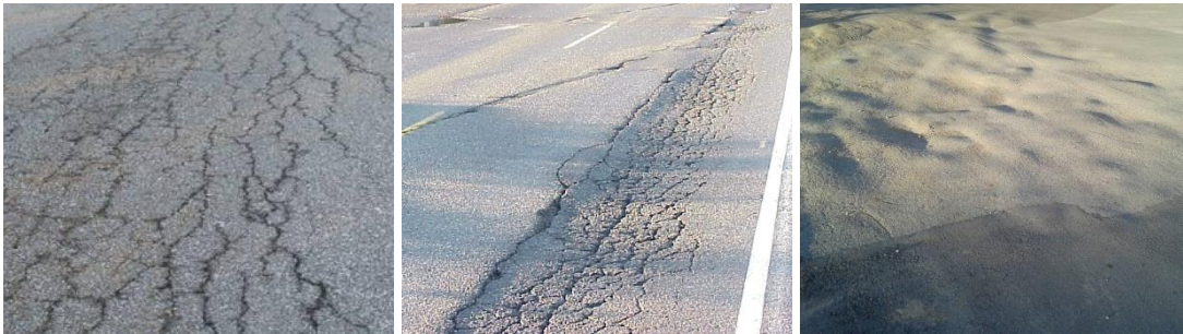
Figure 1 Deterioration of Flexible Pavements
