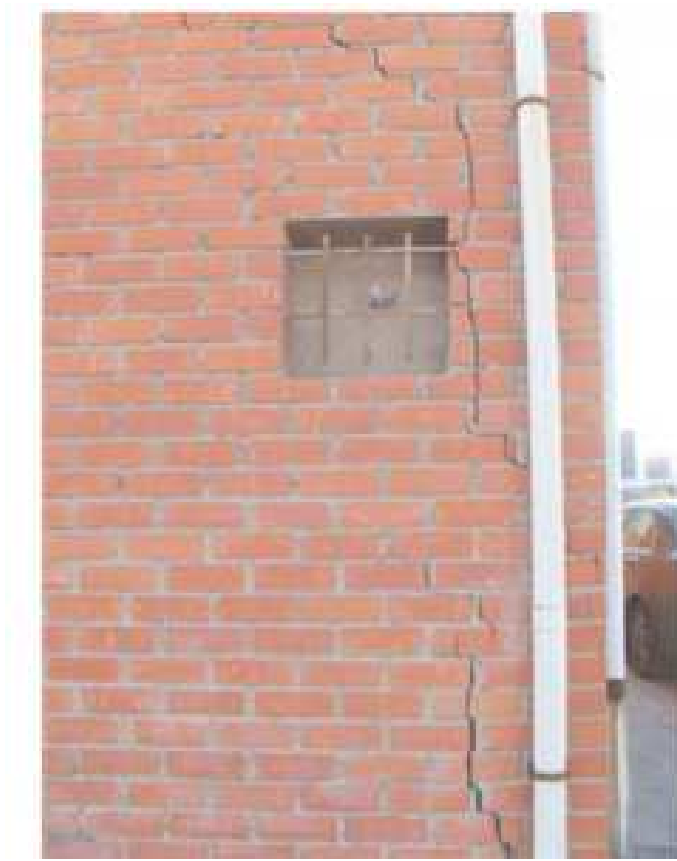
Figure 1.1. Damage to a Building by Swelling of Clays (Yenes et. al., 2012)
