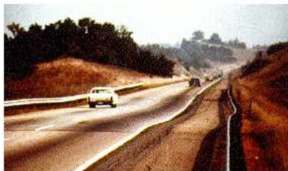
Figure 1.2. A Damaged Pavement Due to Swelling of Soil (DiMillio, 1999)
