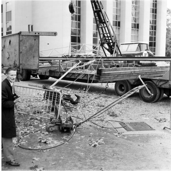
Figure 210. The crane accident while dismantling the mosaic. Source: NATO archives
