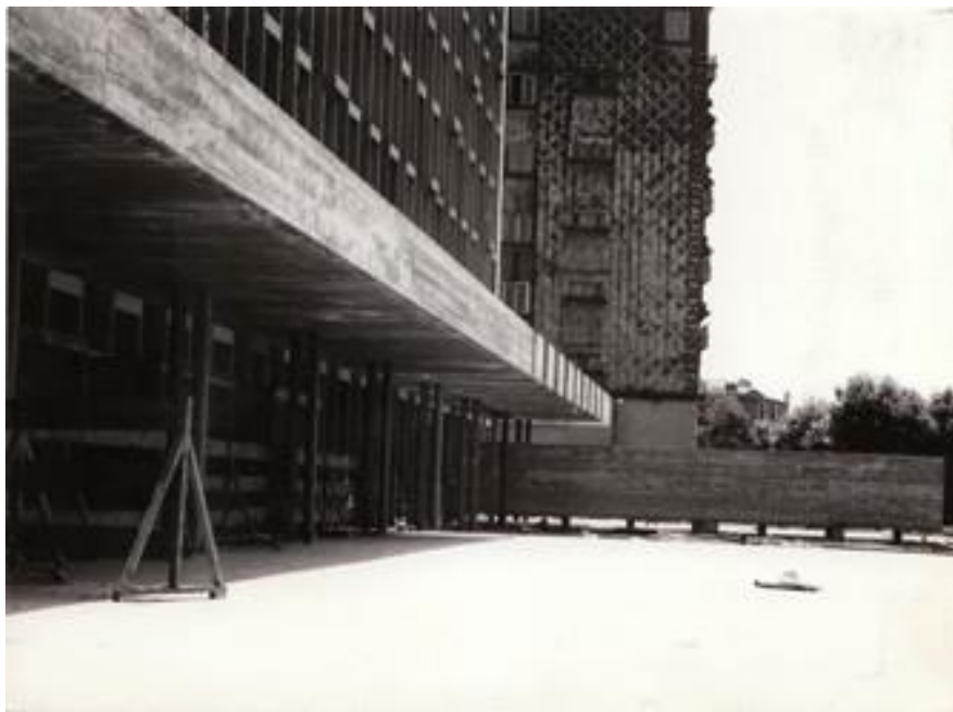
Figure 108. A shot from construction phase of entrance, Atatürk Cultural Center (AKM) Source: SALT Research Archives
