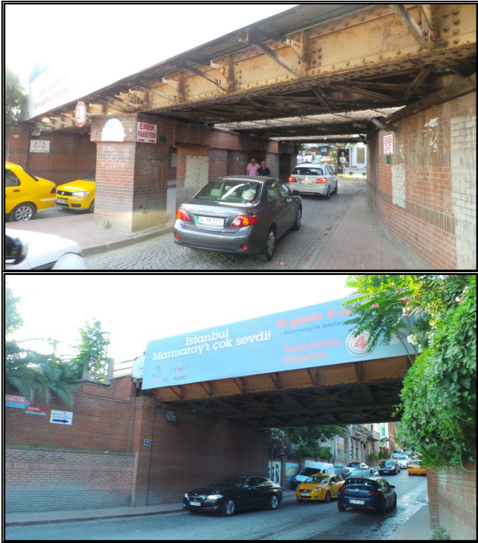
Figure 48: Two different views from the different entrances of car underpasses.
