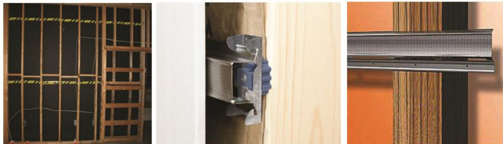
Figure 3.33 Views of a resilient layer applied on wood studs (at the left) and a rubber isolation clip connecting the gypsum board to the wooden frame (at the middle) and a resilient channel applied on a wood stud (at the right).
