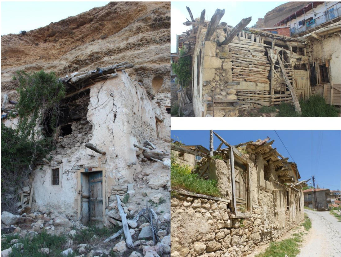
Figure 71: The demolished local traditional buildings in Taşkale Village due to abandonment (author, May 2014)
