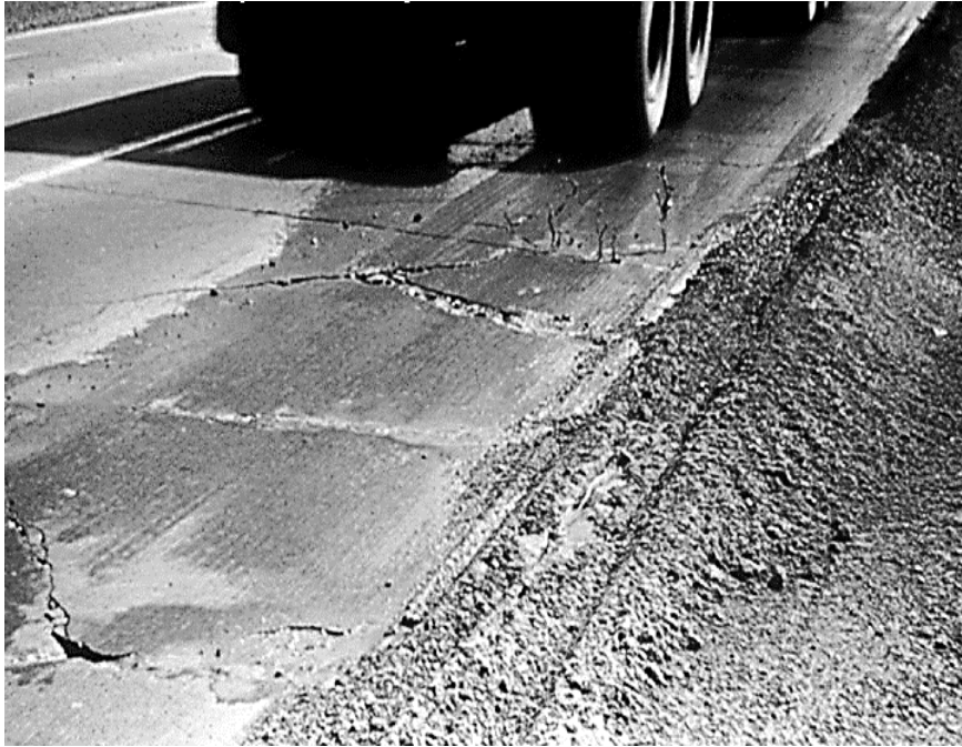
Figure 2.5 Pumping of fines through cracks.
