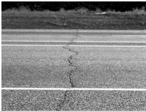
Figure 2.4 An example of thermal cracks in asphalt concrete pavement.
