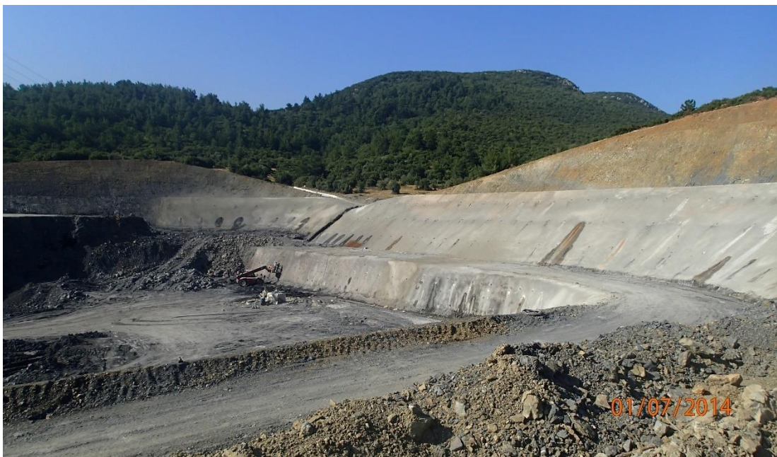
Figure 7. 50 A general view of the forehead slopes after all suggested supports are installed
