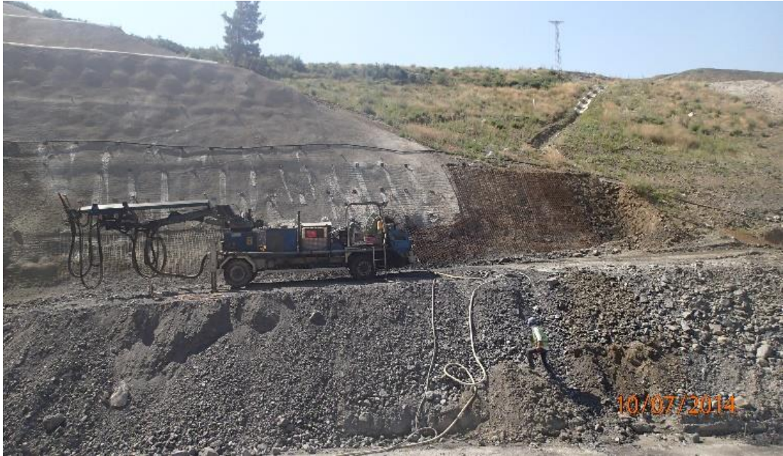
Figure 7. 47 Wire mesh and shotcrete installation for the side slope of the exit portal
