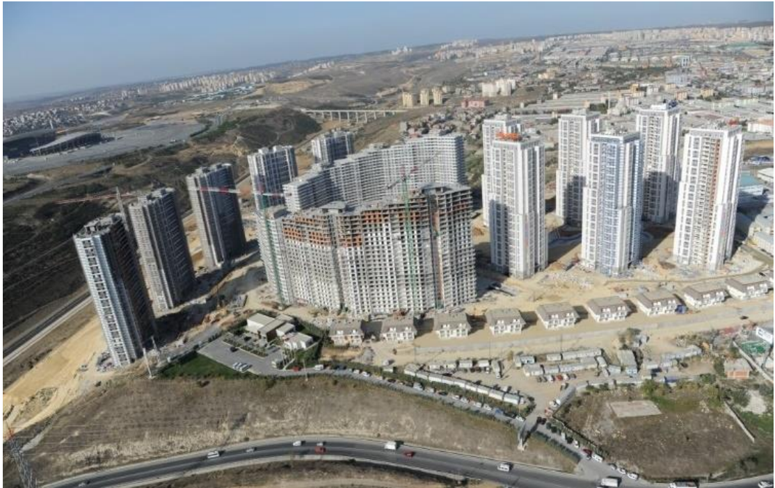
Figure 2-5: Ayazma, after 'urban transformation'. The construction site of 'Ağaoğlu My World Europe' Project. Photo Source: megaprojeleristanbul.com
