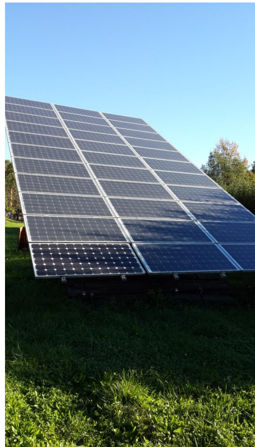
Figure 4.16. PV Panel in Damanhur
