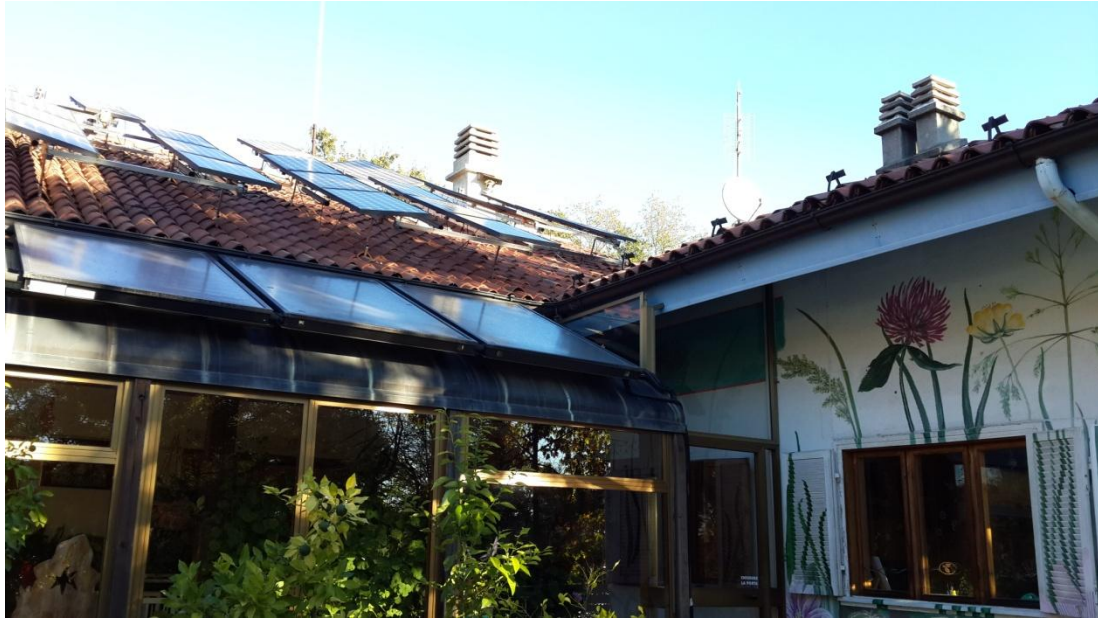
Figure 4.15. Solar Panels on the Roof of a Community House in Damanhur
