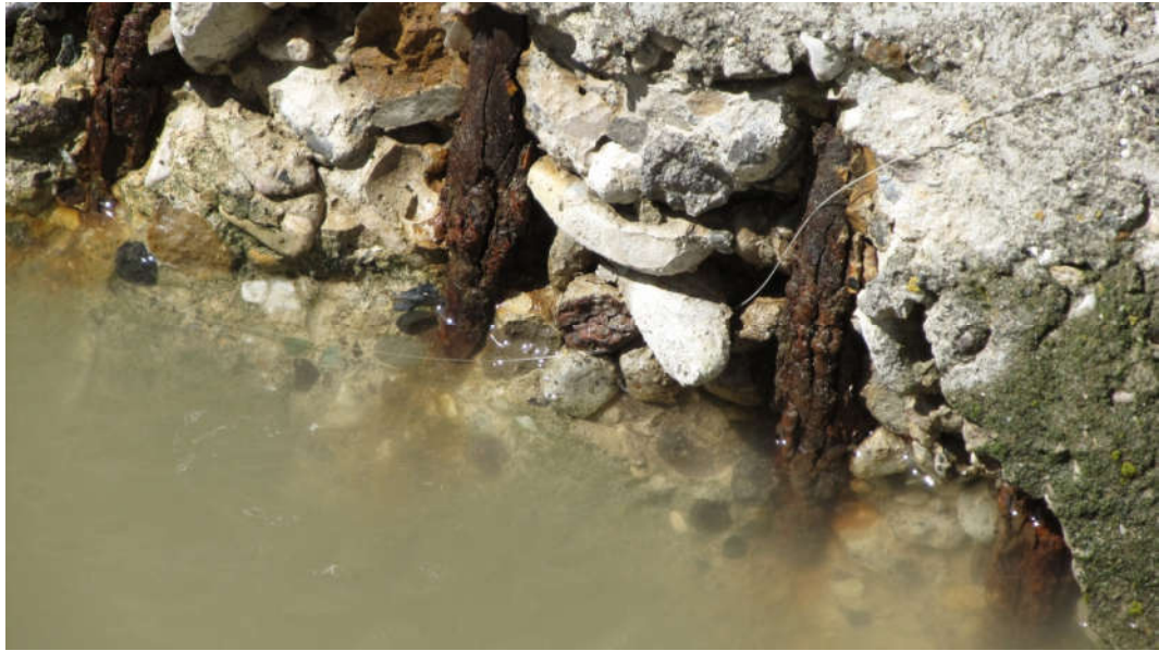
Figure 2.16: Example of Corroded Reinforcement (Özdemir and Topkara, 2015)
