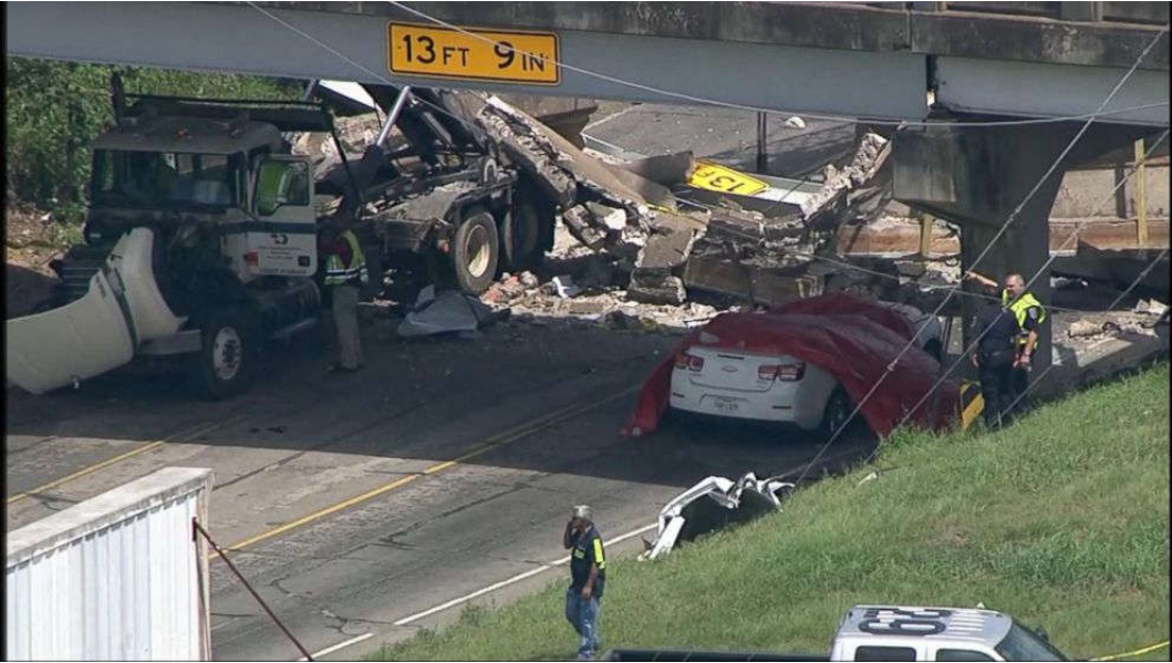
Figure 2.2 Partial Collapse of a Bridge in Texas (ABC News, 2016)
