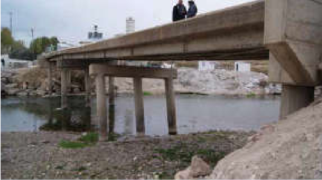
Figure 2.10: Photo of a Bridge after Van Earthquake that was damaged due to a flood few years before (23 Ekim 2011 Mw 7,2 Van Depremi Sismik ve Yapısal Hasara İlişkin Saha Gözlemleri, 2011)
