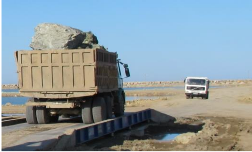
Figure 4.43 Transportation of stones to site by trucks, Retrieved from İbrahim Ahmetoğlu, Project Manager of Cengiz Insaat.
