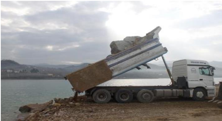
Figure 4.44 Unloading of stones into the sea, Retrieved from İbrahim Ahmetoğlu, Project Manager of Cengiz Insaat.
