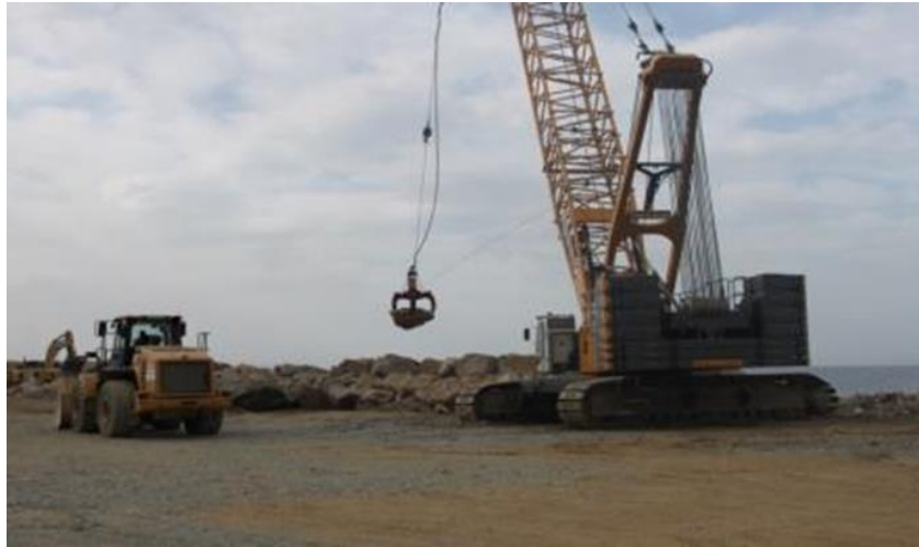
Figure 4.45 Arrangement of rockfill with Crane, Retrieved from İbrahim Ahmetoğlu, Project Manager of Cengiz Insaat.
