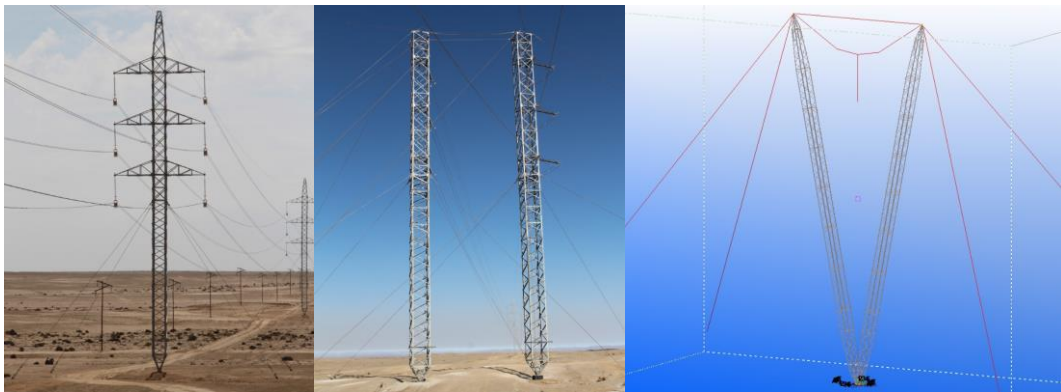
c) Guyed tower examples
