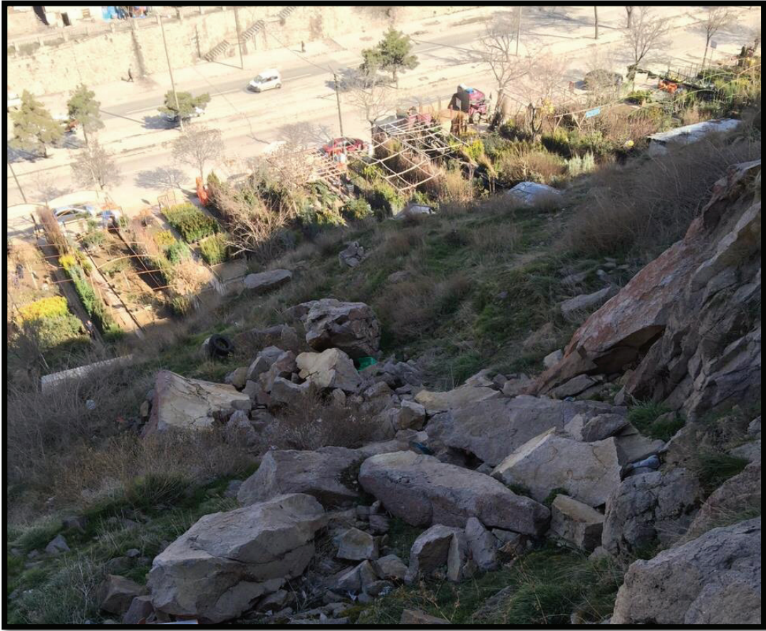
Figure 1.2 Fallen blocks seen in the study area and the floral shops at the bottom of the hill.
