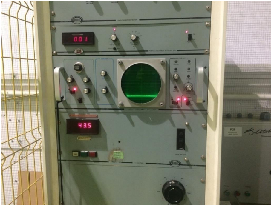
Figure 2-3 Partial discharge test equipment (Biddle 666035-01)
