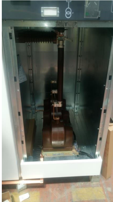
Figure 1-1 A gas insulated MV voltage transformer installed in a 36kV 630A switchgear equipment
