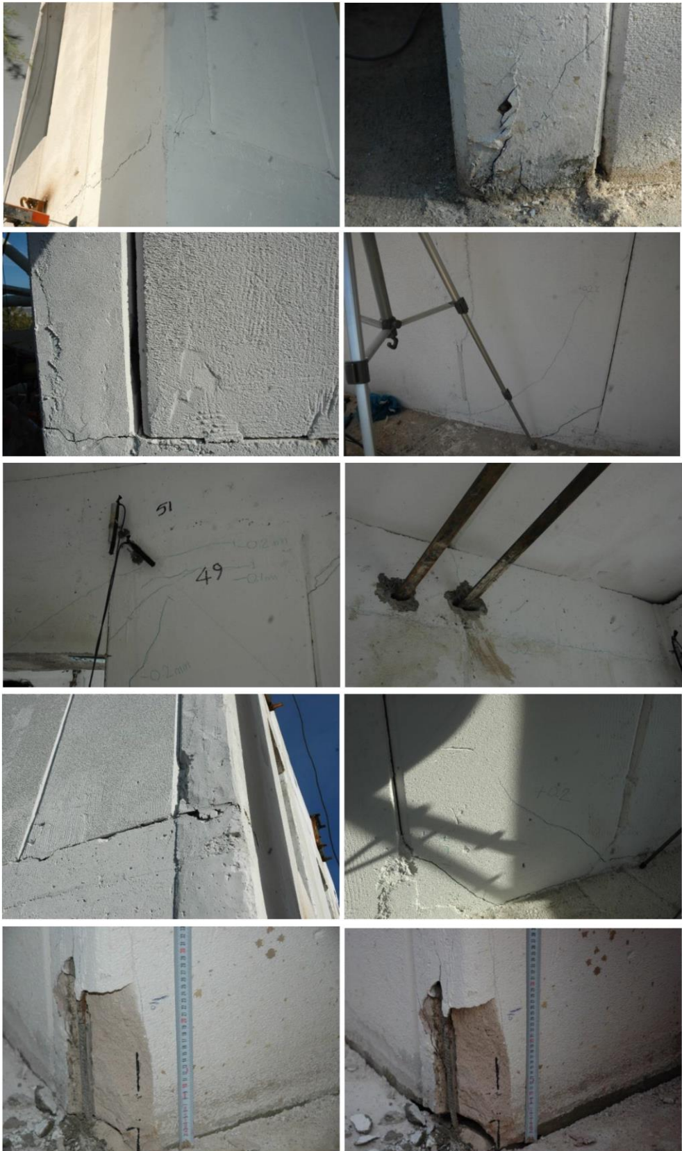
Figure 2.16: Damage Pictures of Project Building
