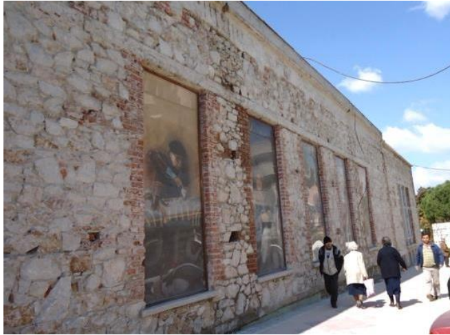
Figure 2. 42. The photo of the east elevation showing the construction technique and material, March 2012
