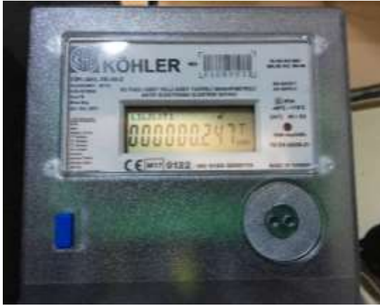
Figure 124. Photograph of electrical meter before oven was turned on
