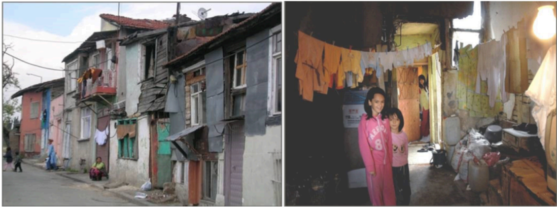
Figure 4-13: Poor conditions of housing buildings in Sulukule before regeneration project Source: http://www.fatih.bel.tr/icerik/1155/neslisah-ve-hatice-sultan-sulukule-mahalleleri-yenileme-projesi/ (Last accessed: 25/04/2018)
