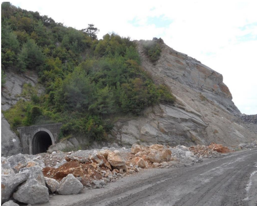
Figure 2. General view of the east portal of the tunnel and the surrounding rock
