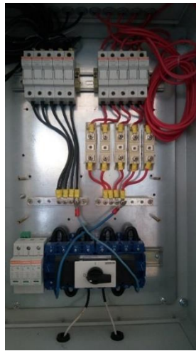
Figure 5-2: Junction box for PV strings
