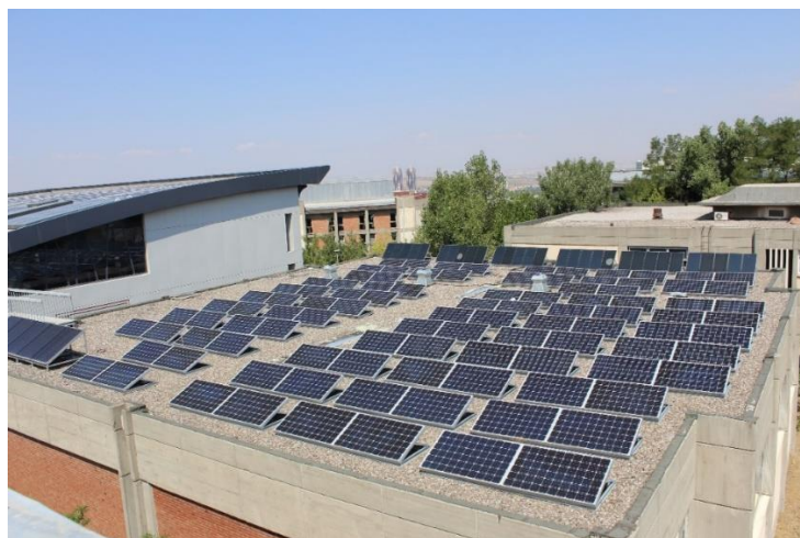
Figure 5-1: PV module installation as power source
