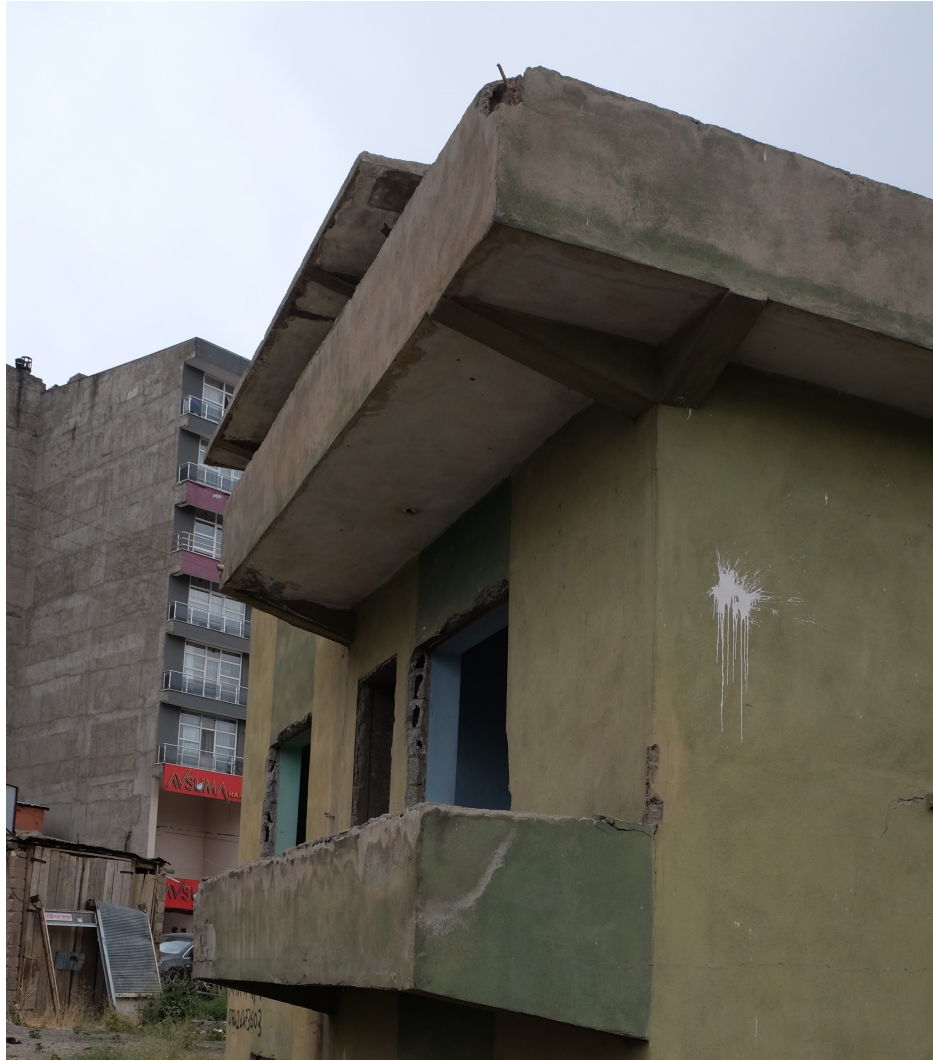
Figure 4.7: Damaged building at the city center (Photo by the author, August, 2017)
