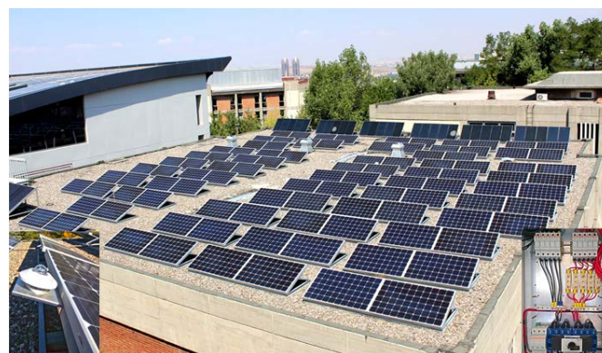
Figure 2. Roof-mounted 23.7 kW at 1000 W/m 2 and 25 °C multi-string PV system containing 95 CSUN250-72M modules (five parallel connected strings of 19 series modules; with adjustable tilt angles of 15°, 30°, 45° and 60°); coordinates 39.890917, 32.782278; five modules in the photograph are idle; terminal box of the system inside the laboratory is shown at the right bottom corner of photograph while the pyranometer is at left bottom corner.
